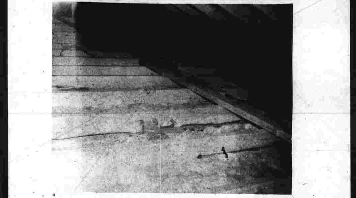
POOR BLANKET INSULATION — PUT IN WHEN THE HOUSE WAS BUILT
